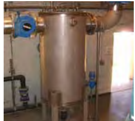
Foam Separator with High and Low Level Switches
