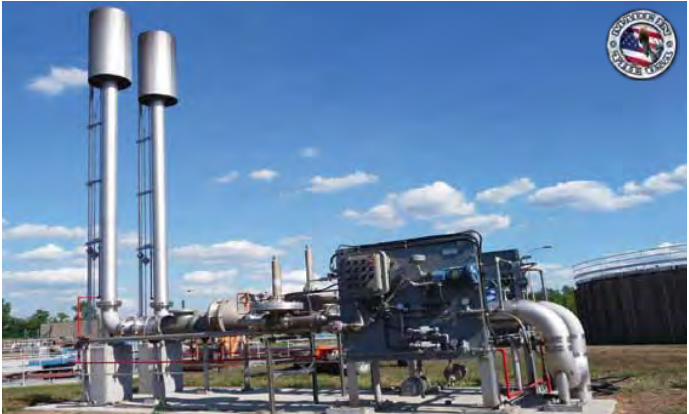
Ground Level Pilot Waste Gas System with two sets of Waste Gas Burners and Control Panels, Regulators & Flame Trap Assemblies
