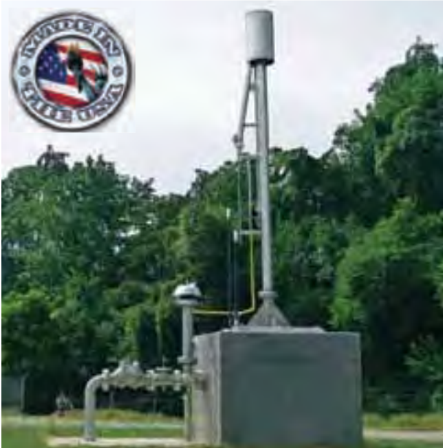
97300 Candlestick Waste Gas Burner with Spark at Tip
