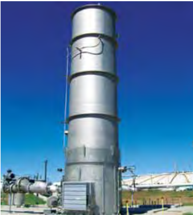
97310 Enclosed Waste Gas Burner with Spark at Tip
