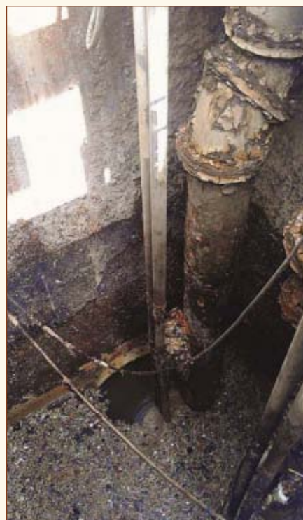
The effects of concrete exposed to high levels of H_2S can be seen in these photos.
