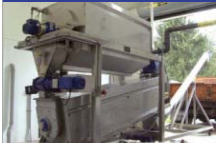
DSP Screw Press Model 3012, NY WWTP
