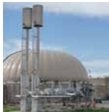
Ground Level Pilot Waste Gas System
