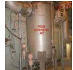
Foam Separator with High and Low Level Switches
