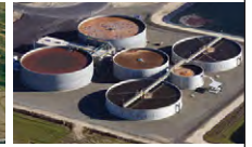
Anoxic & Nitrification Digester Tanks
