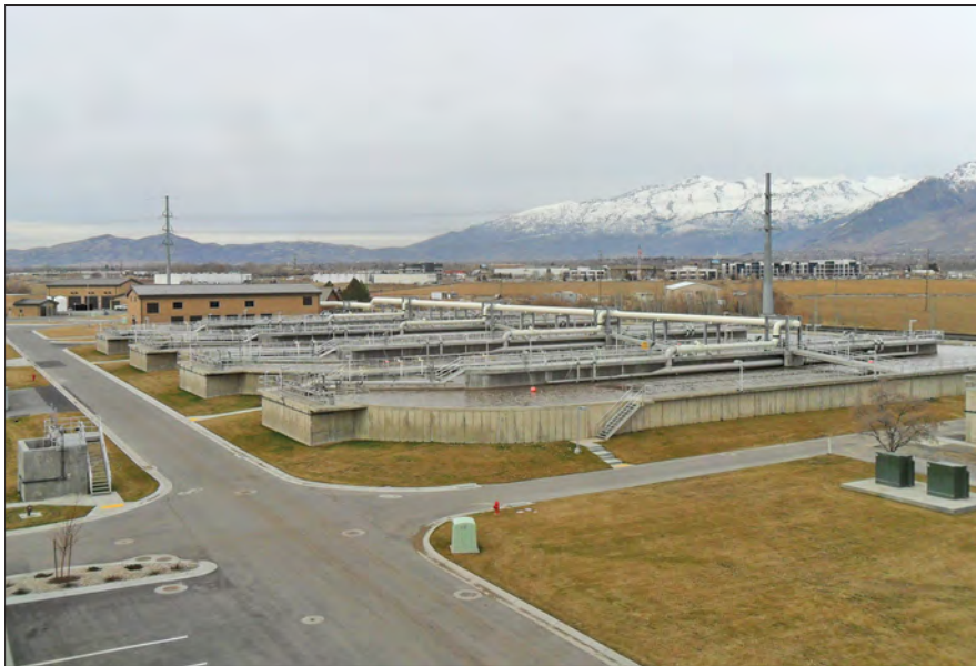
Timpanogos WWT Facility in American Fork Utah where Landia has completed a successful pump and mixer retrofit.
