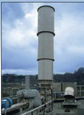
Enclosed Waste Gas Burners
