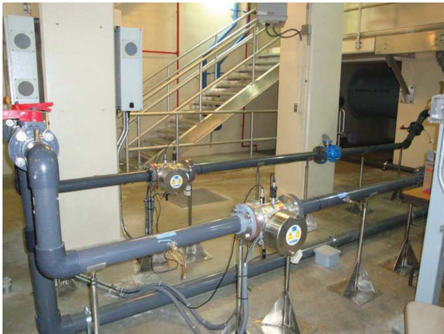
ETS-UV by Neptune Benson UV systems used as part of AOP pilot study
