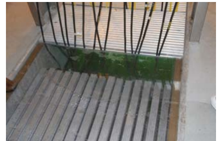
Ultraviolet disinfection of water
