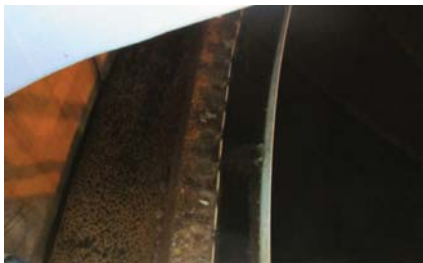
Clear water being collected over weirs at the edges of the secondary clarifier
