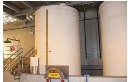
Holding tank for liquid alum used for chemical phosphorus removal
