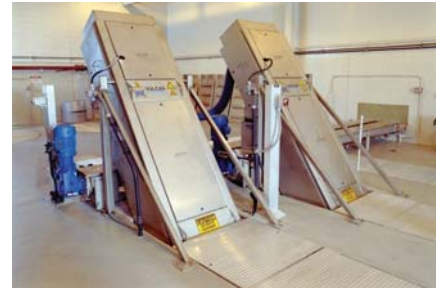
Step Screen in the Headworks Building
