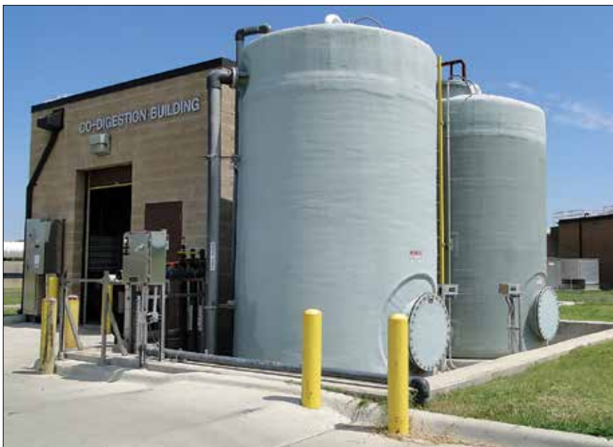
The co-digestion building is where the plant receives industrial wastes. Operators ensure that the wastes do not contain chemicals that would upset the anaerobic digestion process. (Credit: Kristina Twigg)
