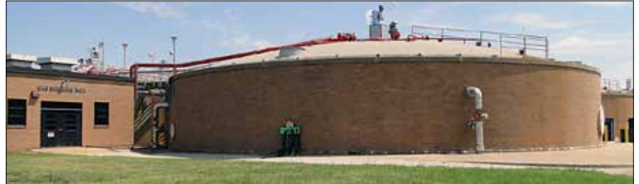
Biogas, used to generate energy via the plant’s turbines, is created in these anaerobic digesters fitted with linear motion mixers. (Credit: Kristina Twigg)
