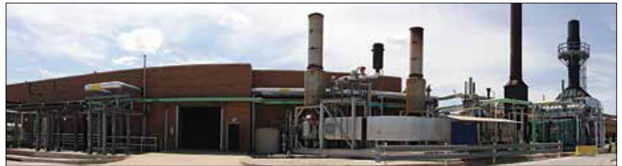
The Village Creek Water Reclamation Facility generates both energy and steam. The steam is used to power two of the plant’s aeration basin blowers. (Credit: Kristina Twigg)
