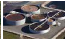
Anoxic & Nitrification Digester Tanks
