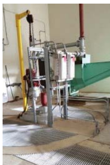
The Sewer Authority's compact PISTA® 360™ Grit Removal System operates in its new headworks building with complete grit pumping and dewatering equipment.
