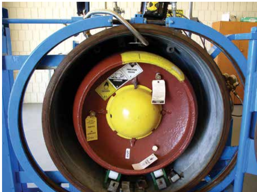
A 1-ton chlorine container is pushed into the secondary containment vessel on rollers. The chlorine transfer hose is attached to the supply valve, pressurized, and tested for any leaks at the hose ends. Then the door is closed, and secured by a clamshell locking mechanism.
