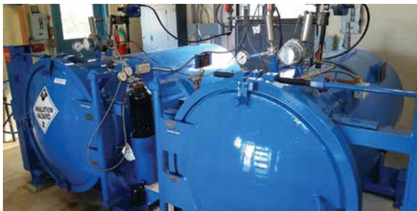
Containment vessels for sulfur dioxide cylinders, stored in a separate building, were similarly installed in 2012, with loader and scale system, and with fail-safe valves and vacuum regulators.
