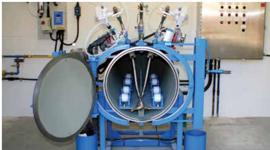
Two 1-ton cylinders of chlorine are stored in a covered building. The ChlorTainer™ containment vessels were installed in 2010 with a loader, scale system, and instrumentation also supplied. A failsafe valve ties into the chlorine sensor. A vacuum regulator can be attached to remove leaking chlorine inside the vessel.
