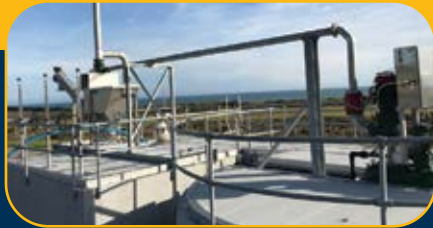
Complete Grit Pumping & Washing
