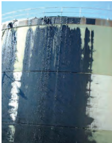
Figure 1: Digester Contents Compromising Roof Structure Integrity
