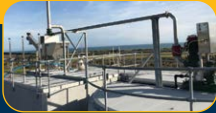
Complete Grit Pumping & Washing
