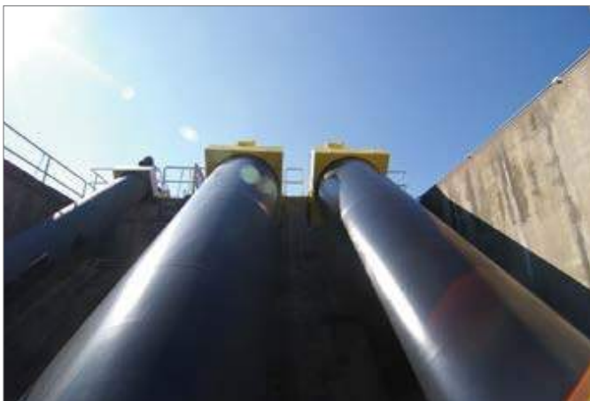
Lakeside's screw pumps in Pennsylvania.
