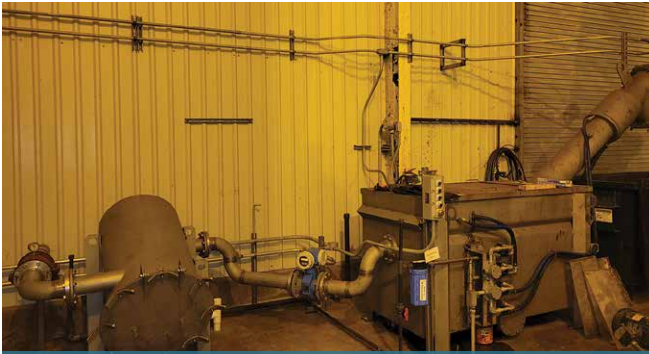
The Lakeside SAP is a small-footprint, pre-engineered, self-contained, fully automated unit.
