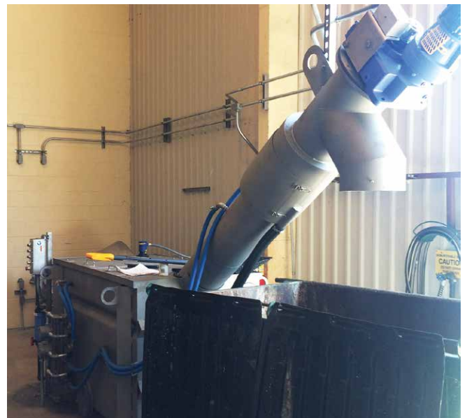
By capturing debris from the septage, damage to downstream equipment such as clogging pumps, is prevented.
