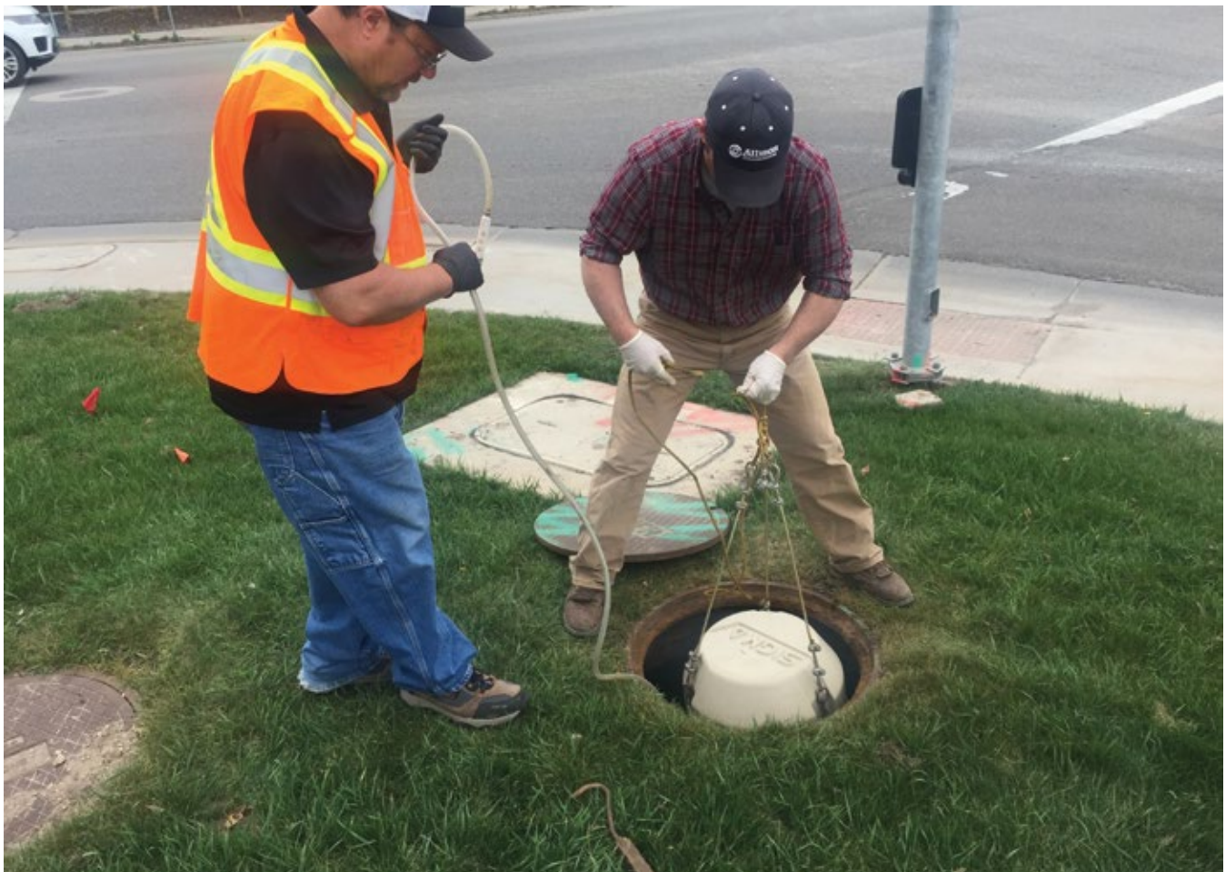
Travis Potter and Chad Burrell from the Snyderville Basin Water Reclamation District install a composite sampler inside one of the interceptors.
