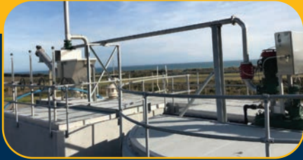
Complete Grit Pumping & Washing
